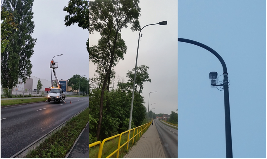
Fig. 6. Mounting measurement equipment along Sporna Street in Bydgoszcz using a bucket truck (Source: [17])
