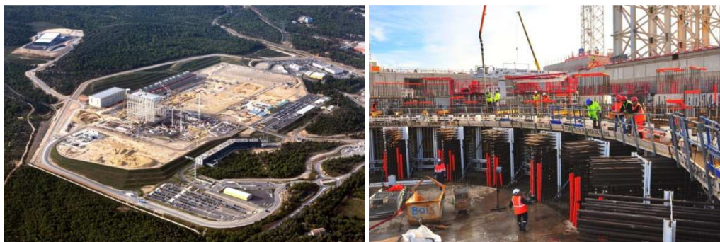
FIG. B-6. Aerial view of the ITER construction site in August 2015 (left). As of 21 October 2015 (right), the 200° segment of the ITER bioshield, the 3.2-metre-thick 'ring' that will surround the machine, was constructed (Photos: ITER).
