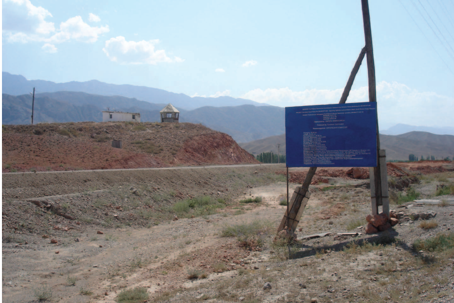
FIGURE 6. START OF THE NEW 23KM BYPASS ROAD AROUND CHORKU AND SURH, FUNDED BY THE EUROPEAN COMMISSION, AUGUST 2008
