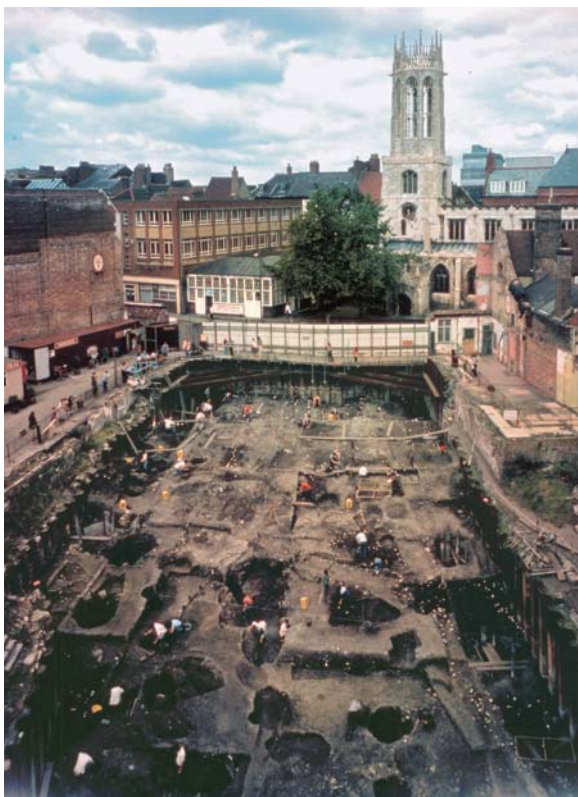
Excavations in progress at Coppergate, before the construction of the shopping complex and Jorvik Viking Centre on the same site.
